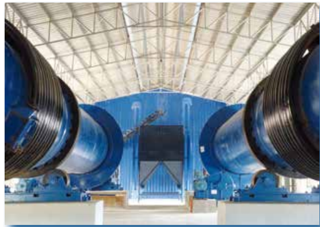
Rotary kilns of the Donau Carbon production plant on the Philippines
